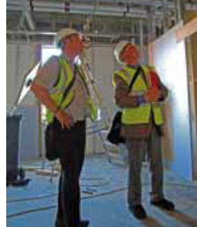
GSS's Shaun Wilson (right) discussing building works in the new isolation ward with Chris Adams of Redworth Associates.
