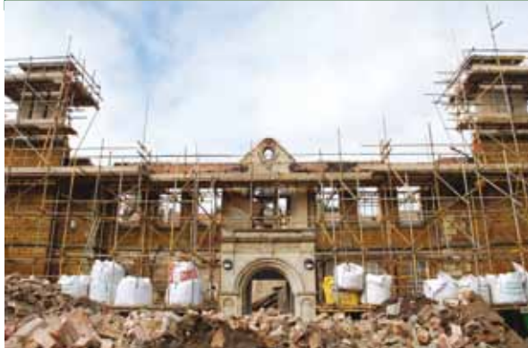
The Manor House after the structure had been made safe following the fire.
